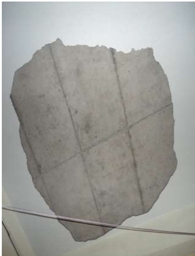
DISTRESS FOUND IN ROOF
