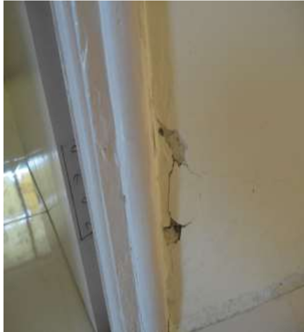
DISTRESS FOUND IN WALL
