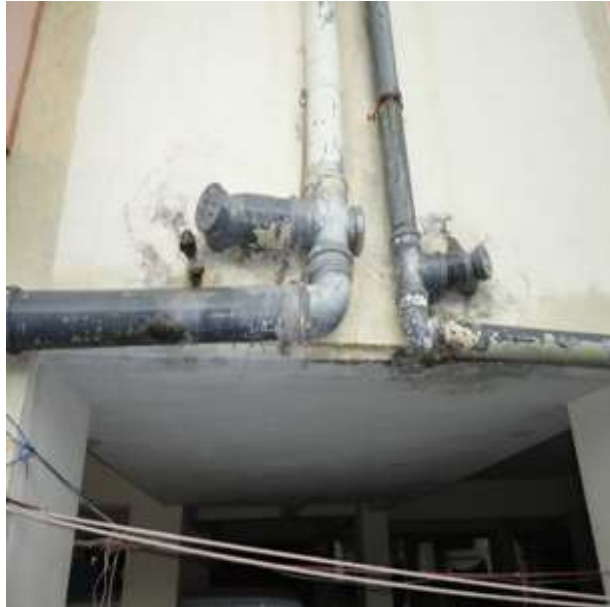
DISTRESS FOUND IN SANITARY SYSTEM
